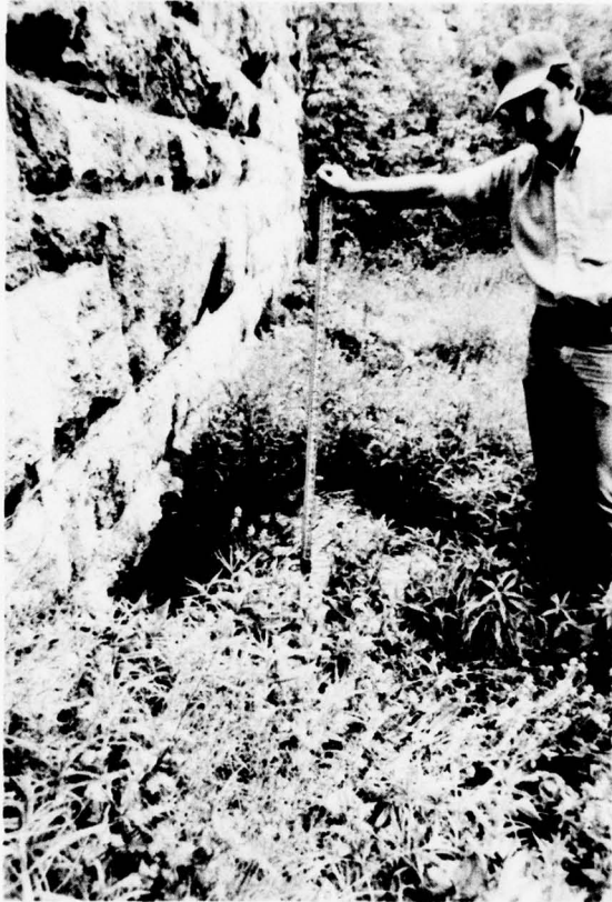
E. Wet Spot Near Downstream Toe of Retaining Wall
